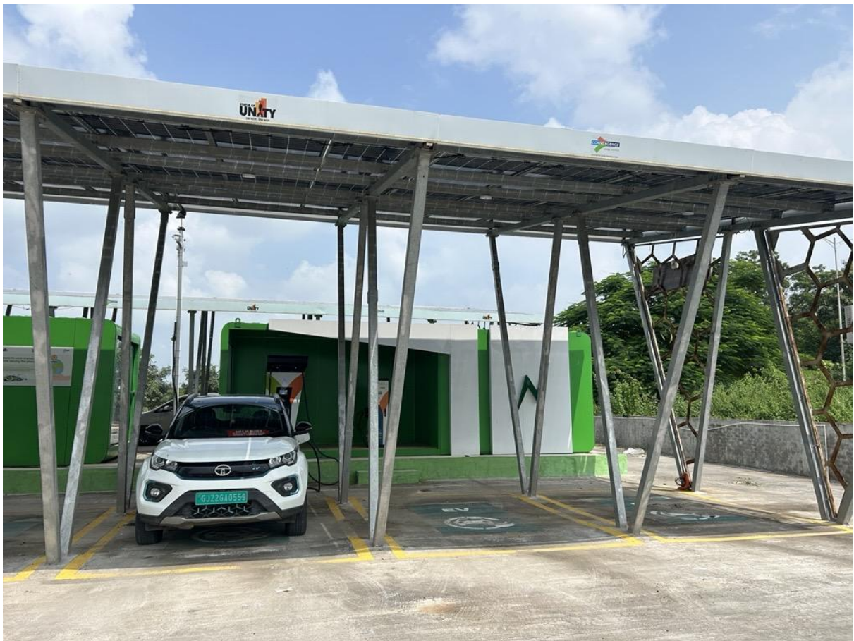
Figure 9: EV charging at SoU site
