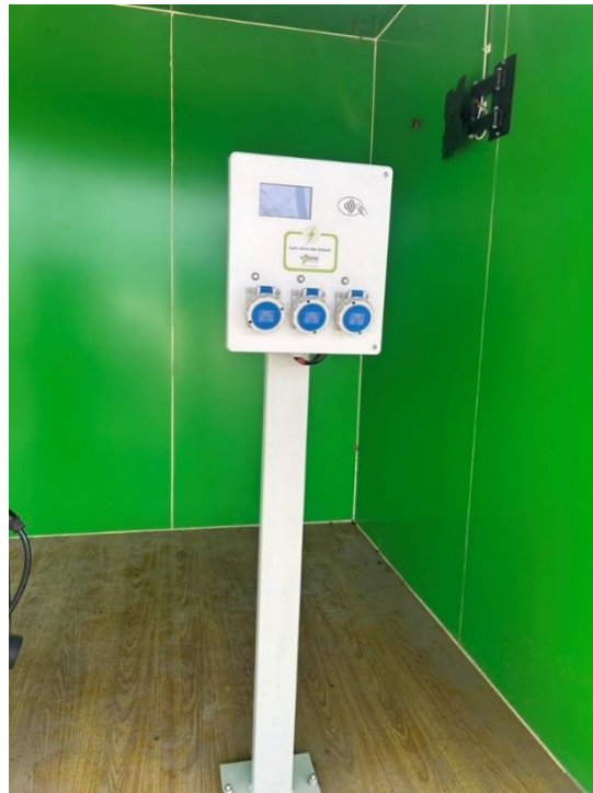
Figure 4: EV Chargers at SOU
